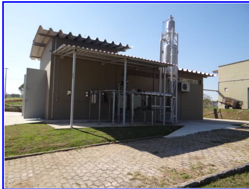
Figure 3. BTBH at IAE's premises
