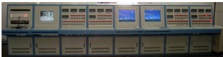
Fig. 4. Photograph of the control panel hardware.
