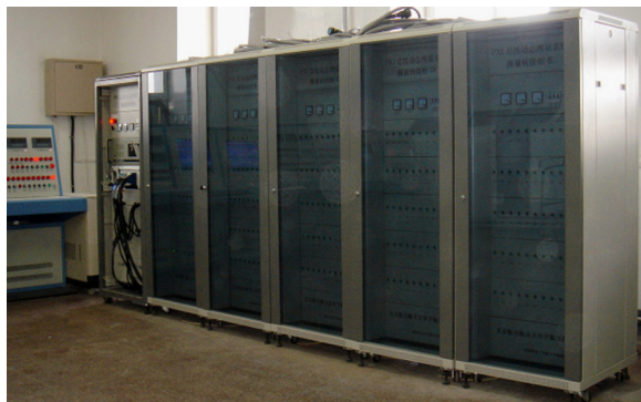
Fig. 3. Cabinets of the measurement system.
